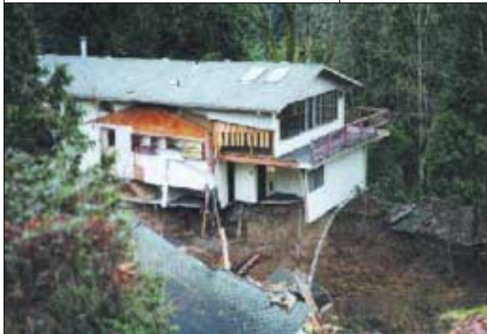
Slope failure claimed 60 homes in Kelso, Washington, in 1998.
